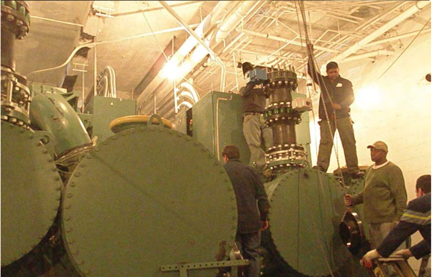
Parts for the chiller room were trucked through Manhattan to get them into The New Yorker.
