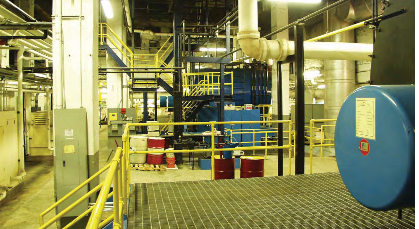
Photos of The New Yorker's updated boiler room.
