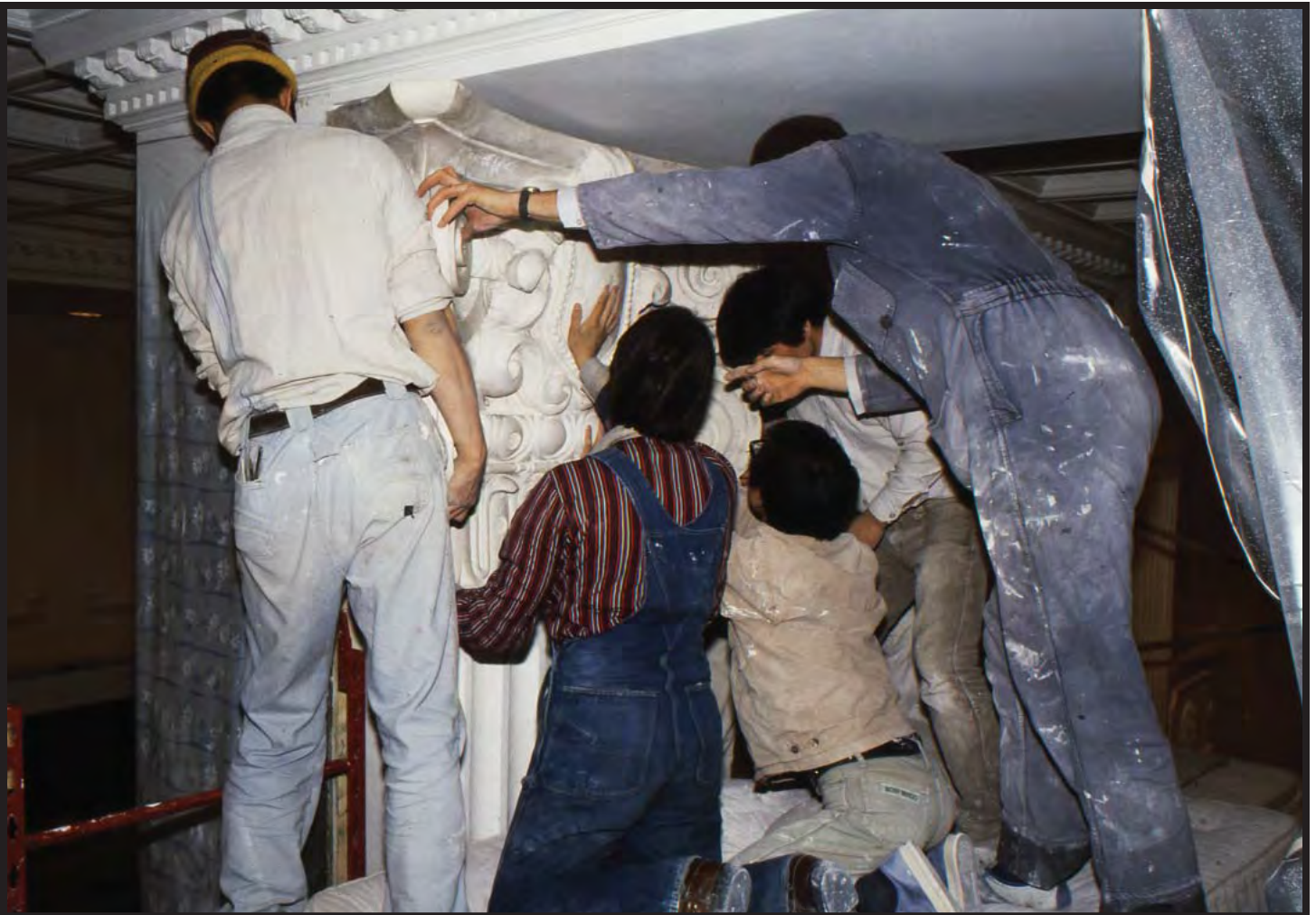
Various photos from the restoration and repair of The New Yorker Hotel under the Unification Church.
