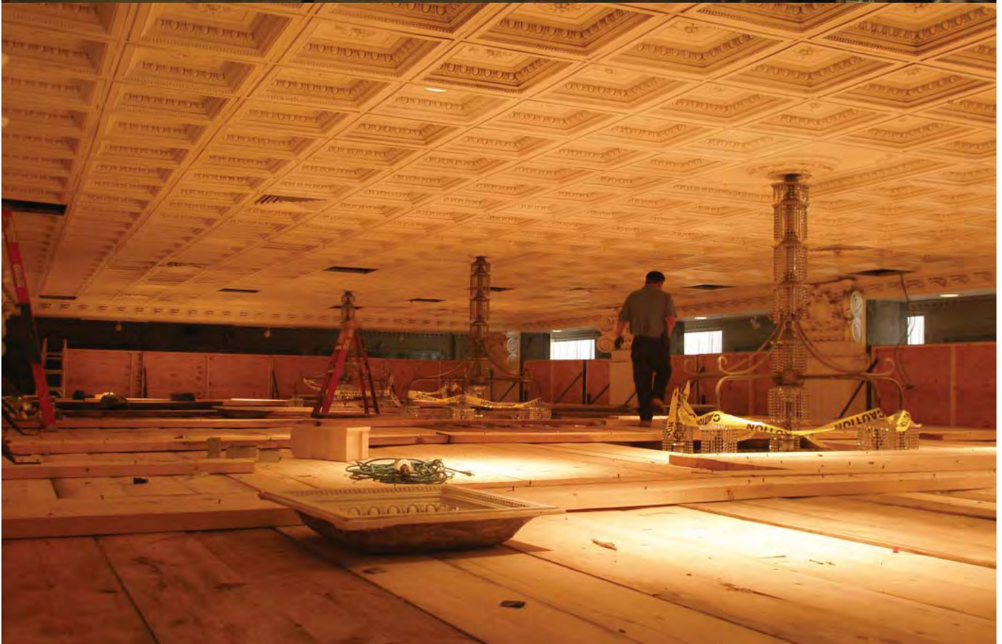
Construction in between the chandeliers and the roof of the lobby. The lobby never closed during the renovation.
