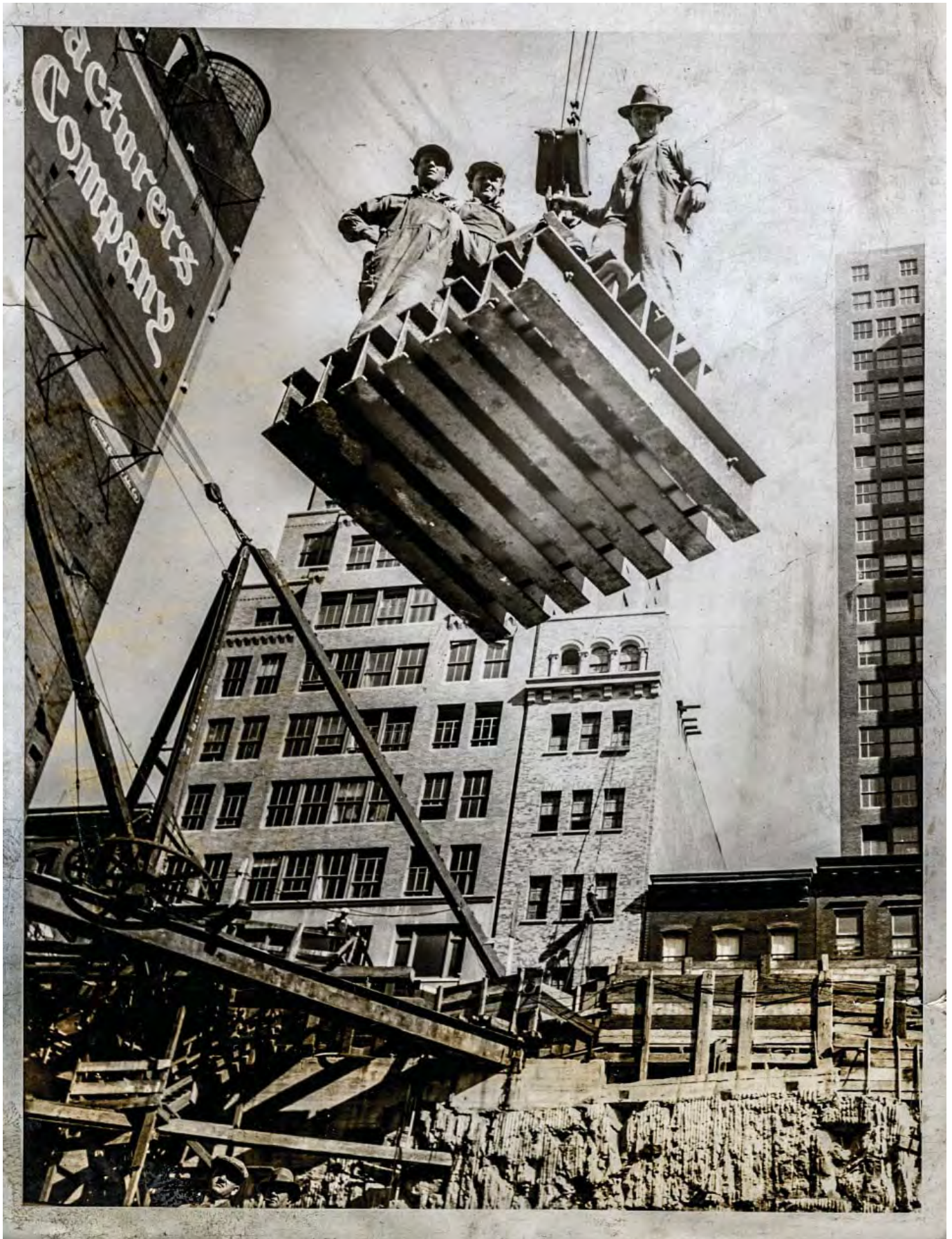
Construction workers during the early stages of construction, riding a footing into place. Workers had to venture 80 feet below street level.
