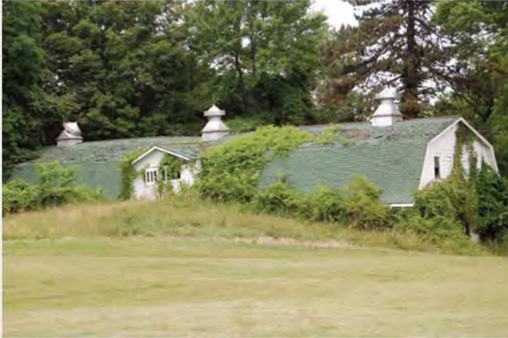
The Potato Barn, where True Father made and repaired fishing nets is in ruins because roof repairs were not done when needed.
