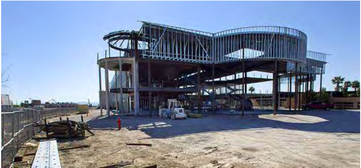
A view of the Peace Palace, a Unification Church convention and training center, under construction at 6590 Bermuda Road, on Monday, April 7, 2014.
