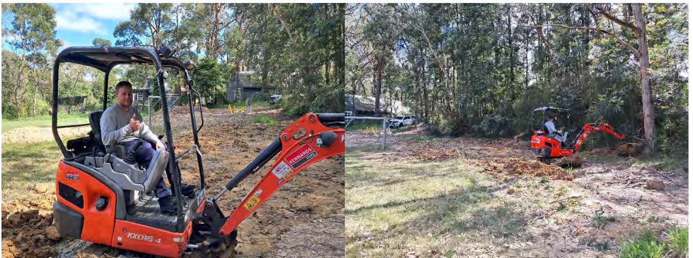
Dean Greenall began working on the repair of the oval, which has been in disrepair since the plumbers laid sewerage pipes down underneath it. Hopefully It can be finished up and green again by the new year.
