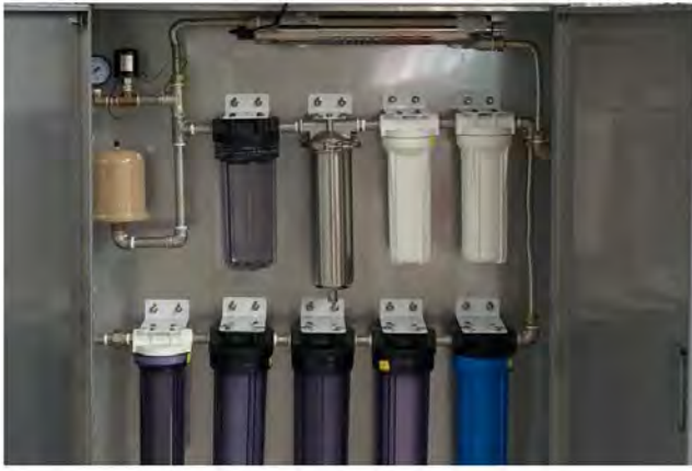
A prototype for purifying water by using a number of different filtration technologies.
