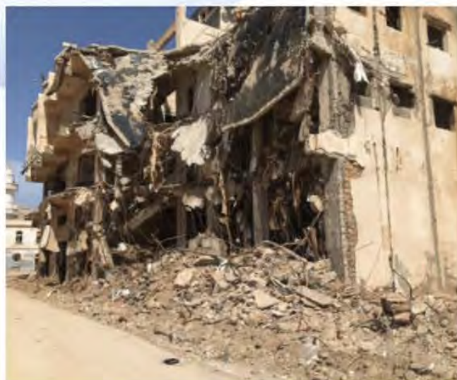
Damage from the flood in Libya. (Photo by Benghazi charity LIFE.)
